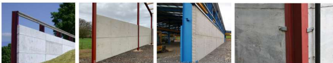
(Left) Bolted to the inside face, (Centre) Slotted in between, (Right) Bolted to outside face
